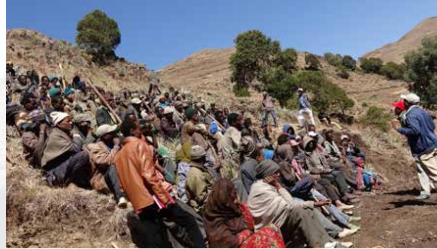
Project teams and communities in Buso watershed, Amhara region, Ethiopia share information on how to construct benches.
