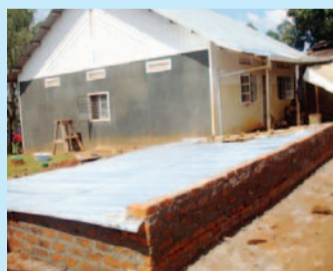
(4) A water tank with a capacity of 30,000 litres
